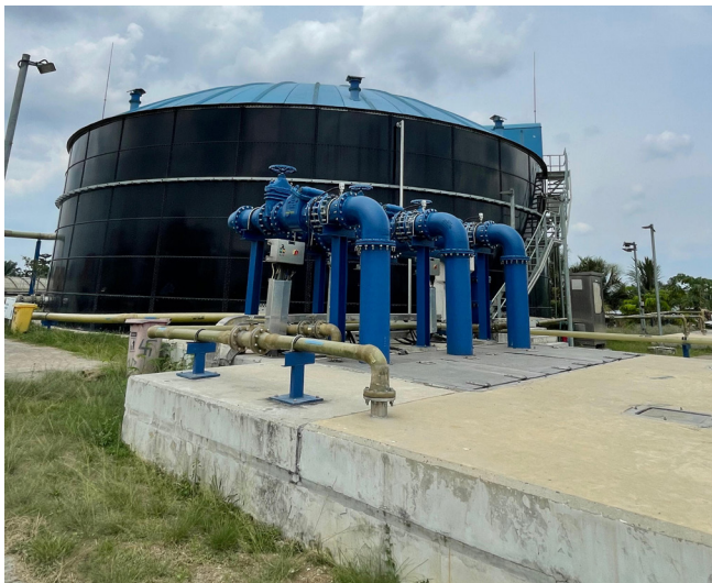
Biological Trickling Filter
